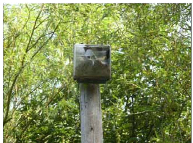
Figure 3.8 – Broken light at Ferndale Road open space
